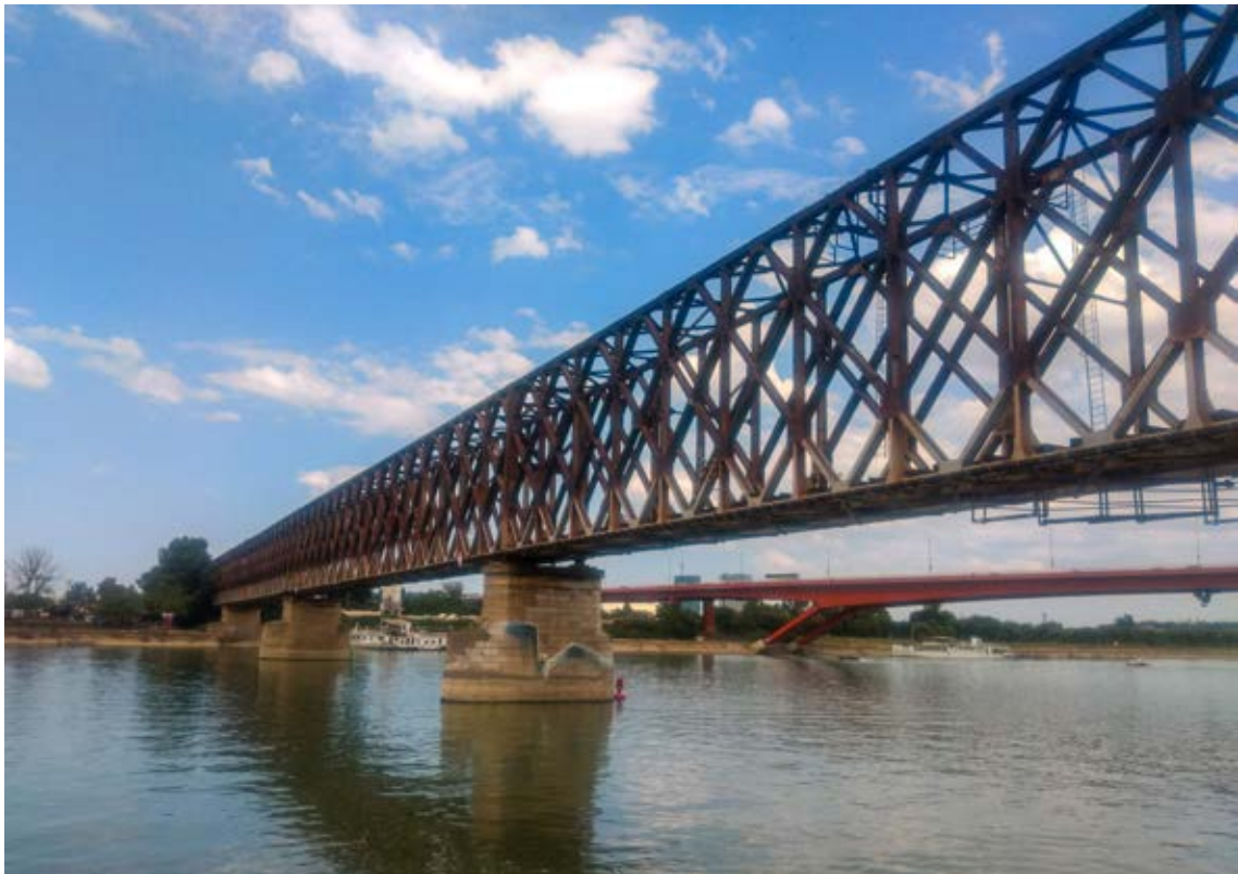
Fig. 7. The Railway Bridge over the Sava river in Belgrade, 2020. (Photo by A. Ilijevski)
